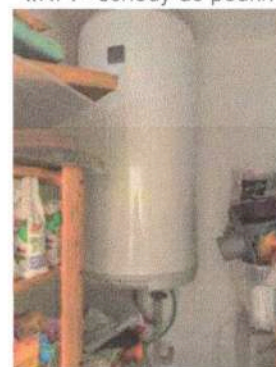
I.NP. - komora/ spiž, el. boiler
